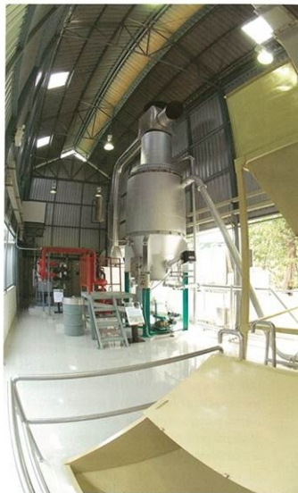
The rice-husk furnace and the absorption chiller air-cooling system
