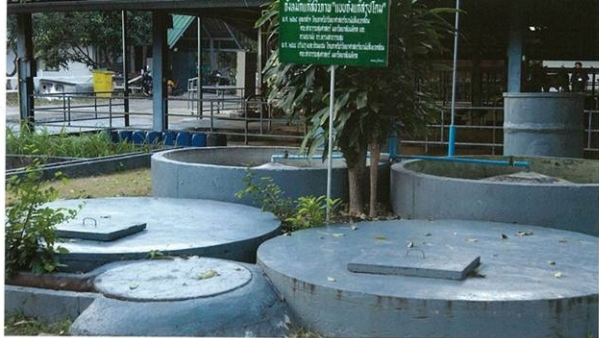
Biogas digester tank in front of the old dairy cow barn
